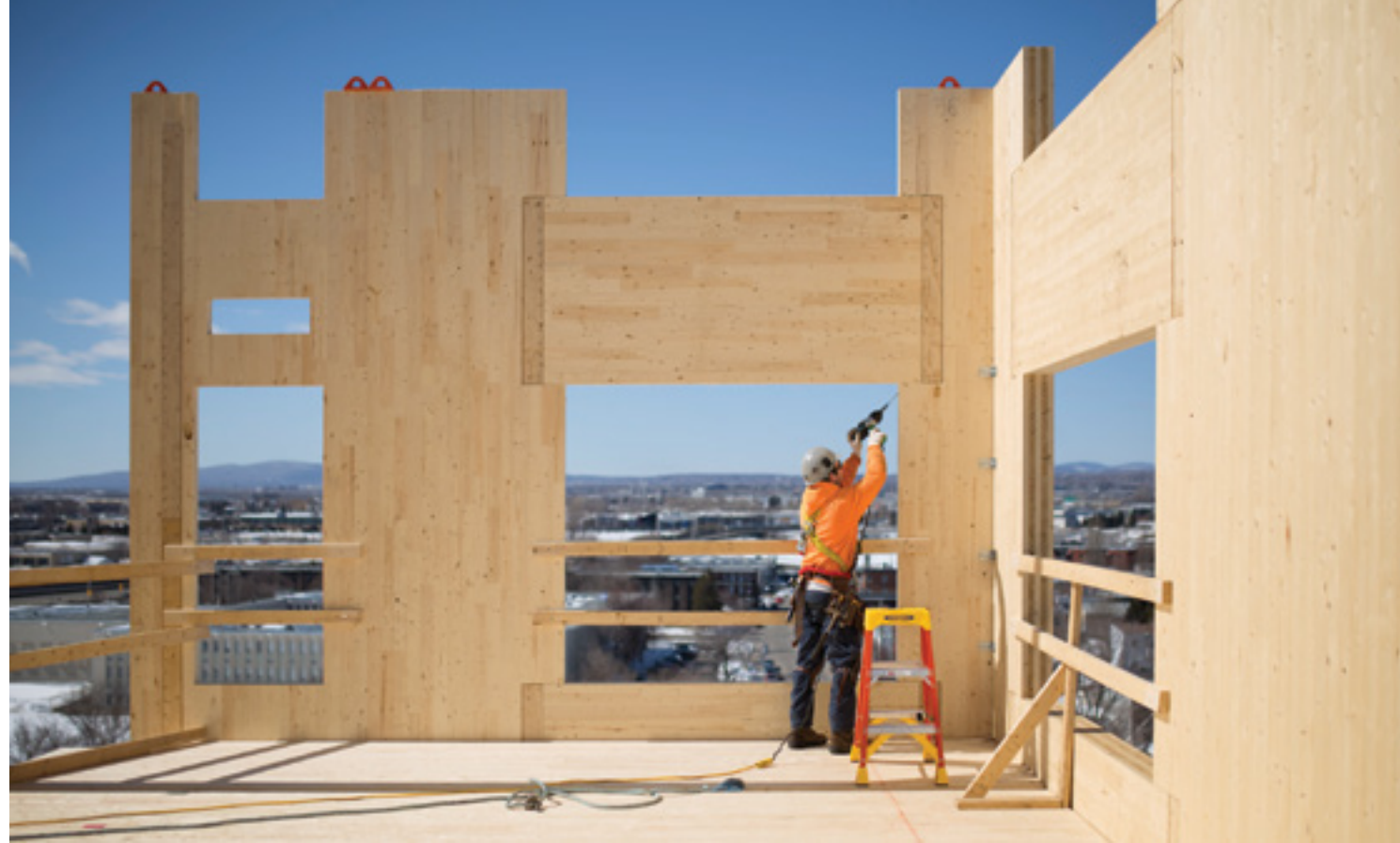
Construction of the 14-floor Origine, in Québec, which is the tallest all-wood condominium building in North America.
