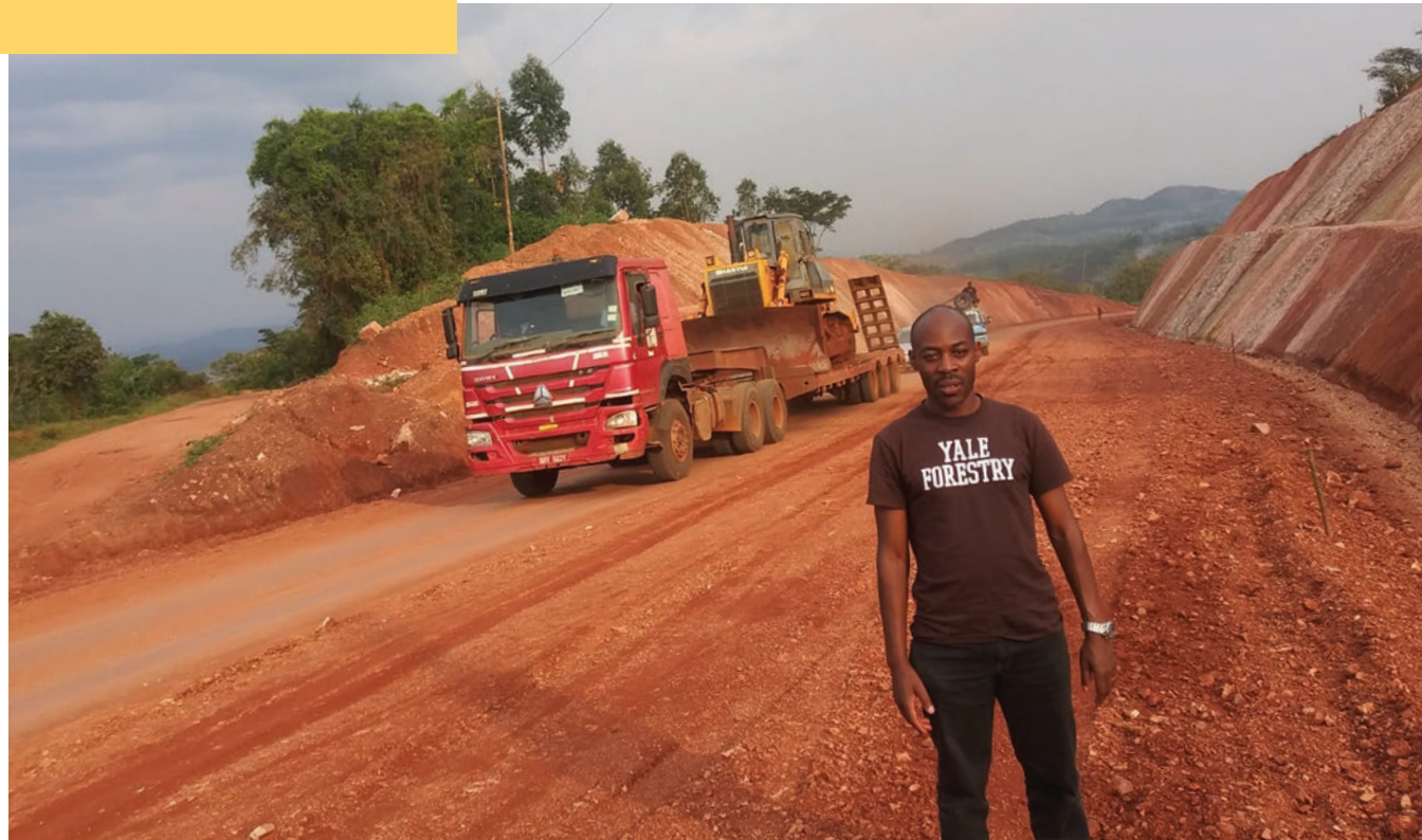
Paul Hatanga stands alongside a new road in western Uganda this summer.
